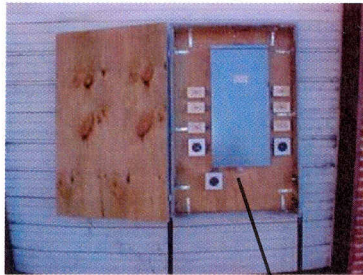
Typical 200 amp River fest load center (for electrical distribution)
